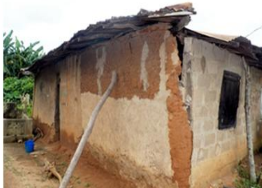
Fig. 4: A cracked and dilapidated settlement in Olapeleke
