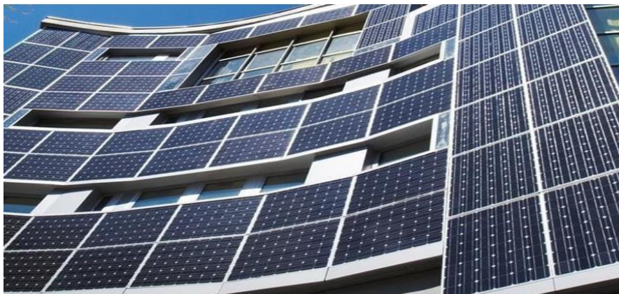
Fig 4. Building Integrated PV
