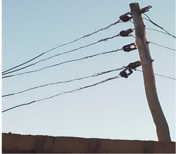
Figure 16. Undersized 415V line conductor and
