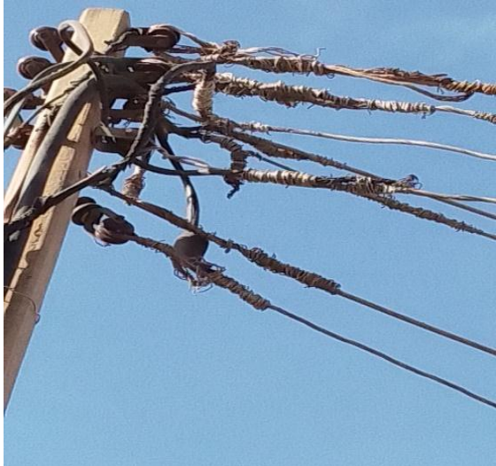
Figure 15. Substandard cable jointing due lack of using line tap and proper cable arrangement. Wooden pole.
