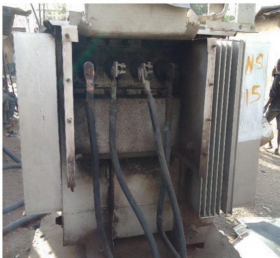
Figure 9. Unprotected 11/0.415KV sub station.
