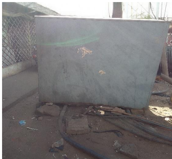
Figure 10. Exposed underground cables
