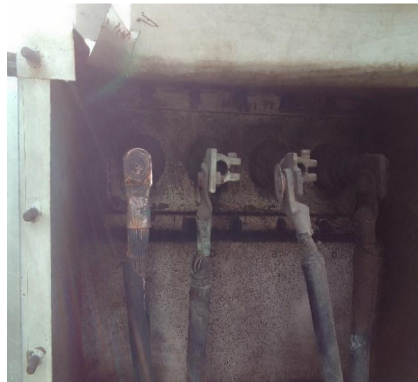
Figure 8. 415V up riser cable insulation break down due to partial contact/over load
