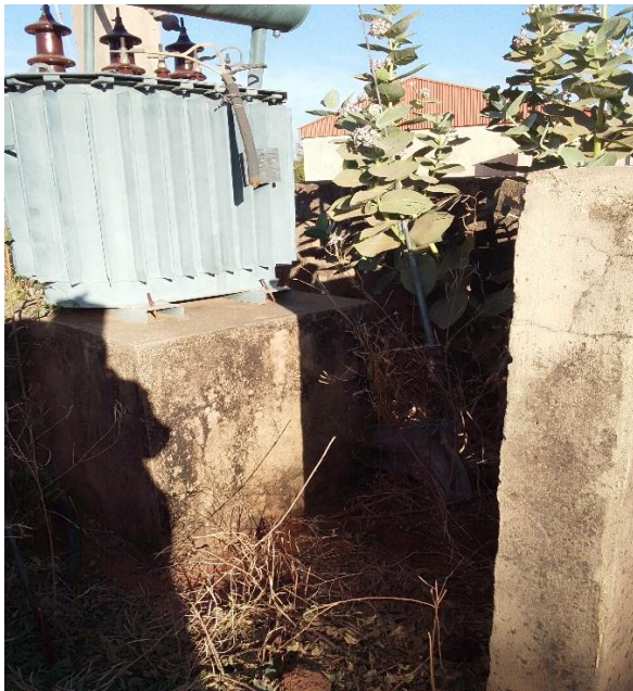
Figure 17. Vandalized 415volt substation.
