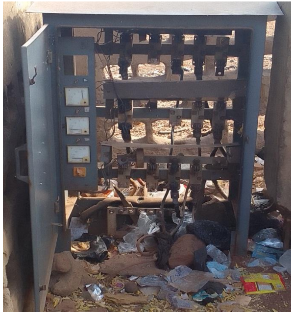
18. Substandard 415volt bus bar
