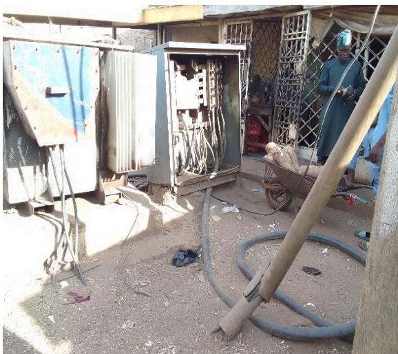
Figure 7. Exposed and unfenced 415V Bus bar in service.
