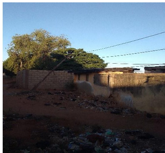
Figure 14. Low tension pole along with line Inclined at 45° on a tree around a residential Building.
