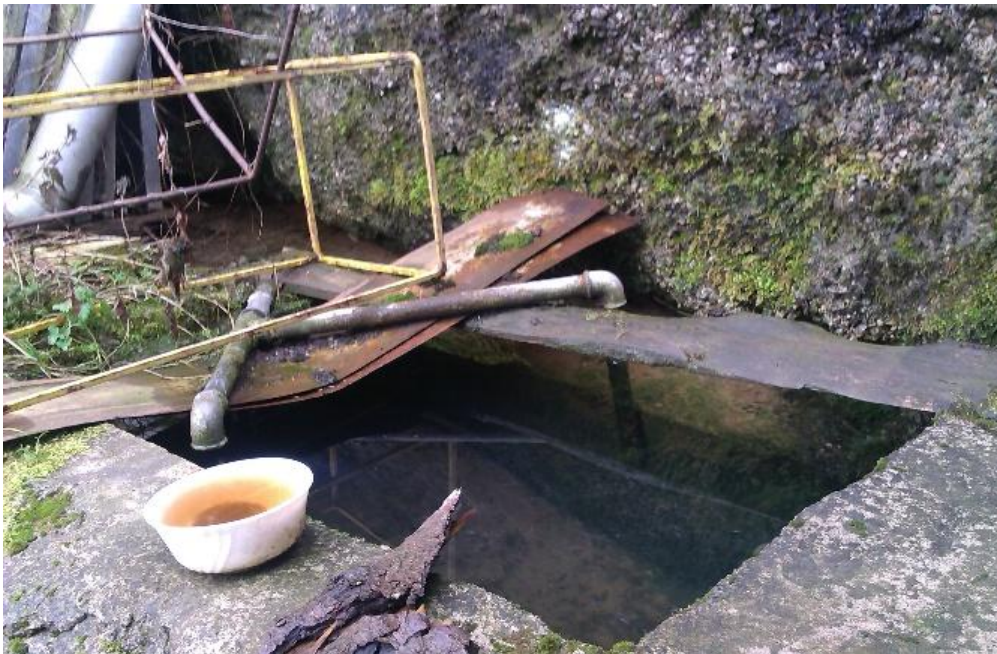
Figure 3. Local drainage/water system element at the site (from the design documentation).
