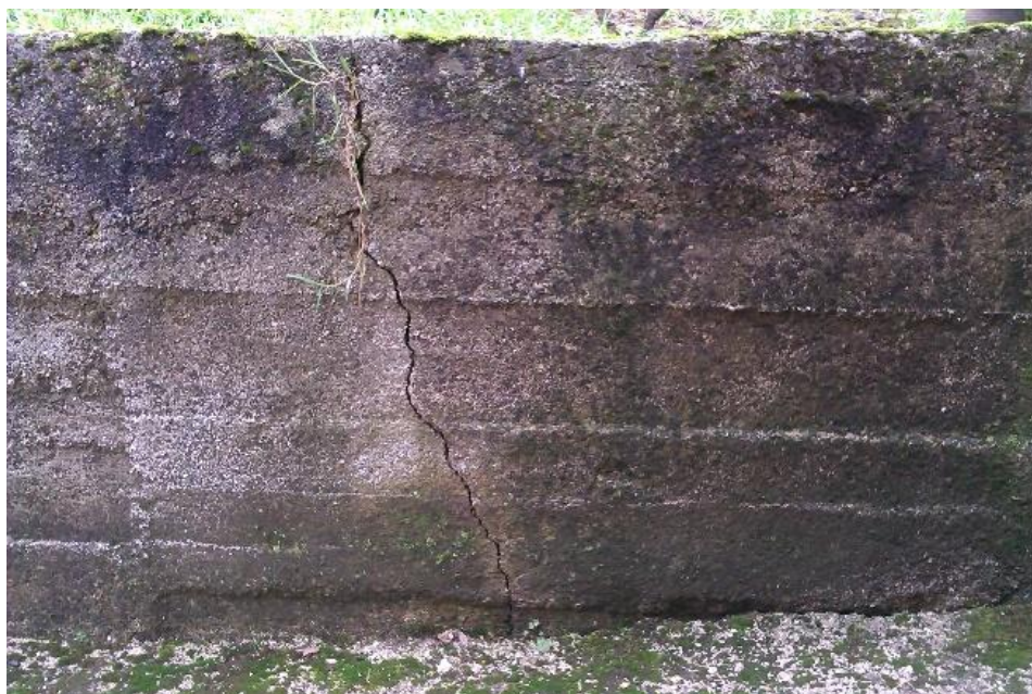
Figure 6. Cracks and damage to the existing retaining wall (from the design documentation).
