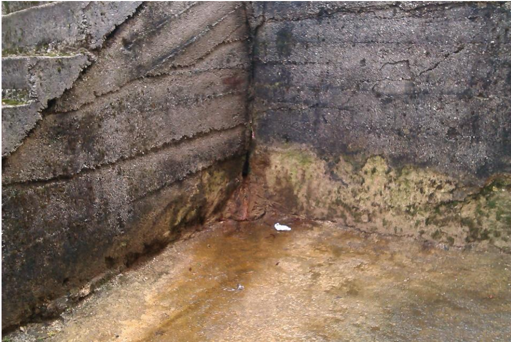
Figure 2. Water observed adjacent to an existing structure at the site (from the design documentation).
